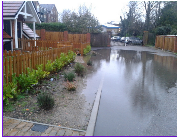
Fig 7. flooding to highway and property due to pumping station failure
