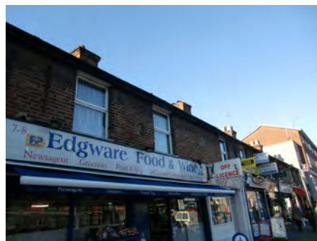
Picture 5.26 Fascia board for nos. 7-8 High Street which cuts across the two units, detracting from the regularity of the terrace
