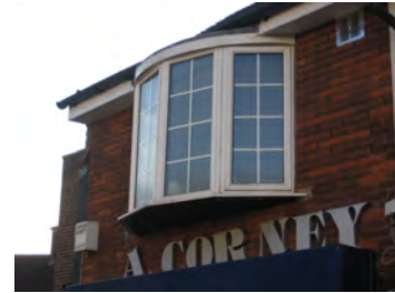
Picture 5.47 Bay window to no. 81 High Street. Although it could benefit from replacement with the use of timber to create more delicate transoms and mullions
