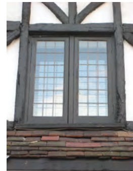
Picture 5.49 Good timber casement led light window to nos. 97-101 High Street, Edgware
