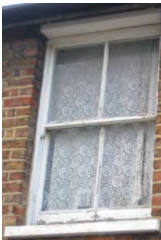
Picture 5.48 The original two over two pane timber sash window on the first floor of the Whitchurch Lane terrace
