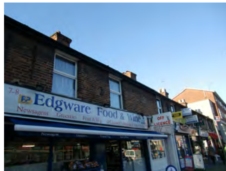
Picture 5.26 Fascia board for nos. 7-8 High Street which cuts across the two units, detracting from the regularity of the terrace
