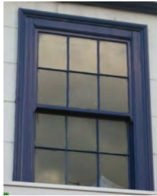
Picture 5.46 Vertical emphasis to first floor windows with this one being a double hung 6 over 6 pane sash window
