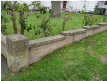
Picture 4.96 Original low boundary treatment to 5 Kerry Avenue of Dunbrik, typical of those original boundary treatments within the Conservation Area
