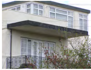
Picture 4.48 First floor balcony to 8 Valencia Road
