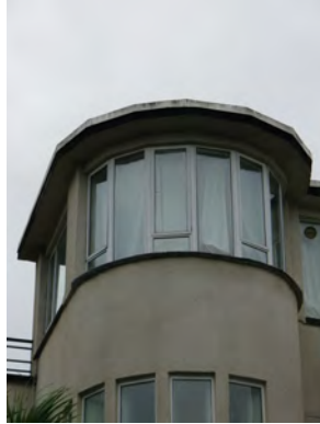
Picture 4.84 Replacement windows here detract from the intended delicate nature of these windows and strong geometrical lines of the building
