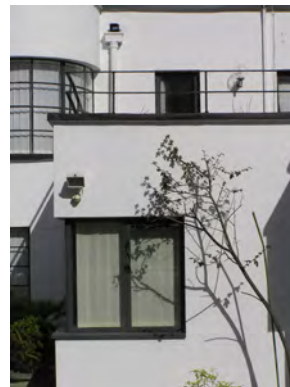
Picture 4.63 Flat roof with sundeck feature on 6 Kerry Avenue, key to its Modernist Design
