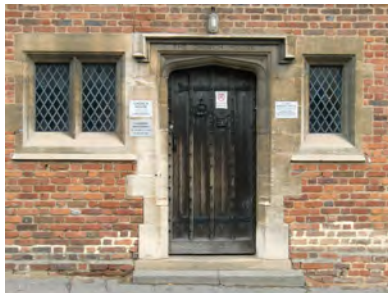
Picture 3.66 Stone and timber Tudor revival style details to the windows and door of Church House, Old Church Lane
