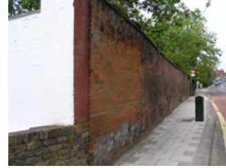
Picture 2.5 Locally listed historic brick wall fronting public highway, lower reaches of Stanmore Hill
