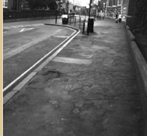
Poor quality street surface, in front of Speech Room, Grove Hill
