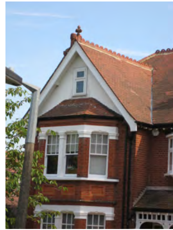
Picture 4.30 Decorative clay pinnacles and ridge tiles, as well as recessed brick aprons
