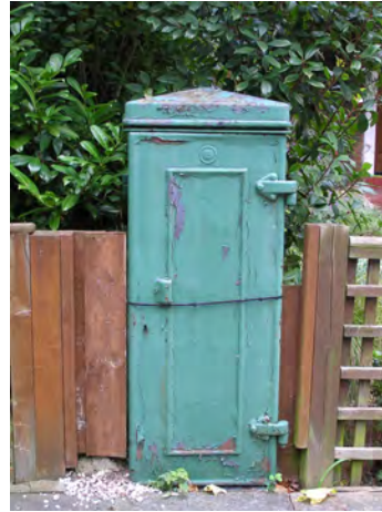
Picture 8.41 Cast iron electric supply feeder
