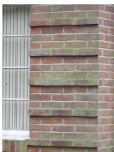
Picture 9.25 Projecting bricks
