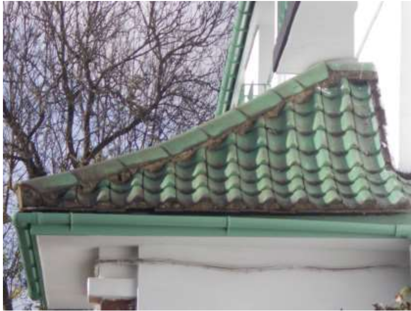
Figure 48: Typical pan tiled hipped roofs of Capel Gardens are part of the colonial/hacienda style
