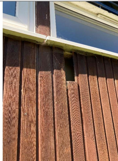
Photograph 3. PRF in the wooden boarding of the east side of the main building.
