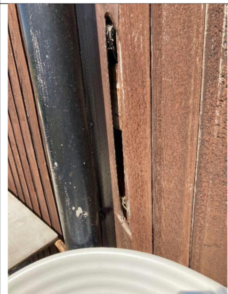
Photograph 4. PRF in wooden paneling of south side of main building.
